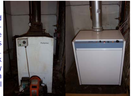
Old oil fired boiler New gas fired boiler
